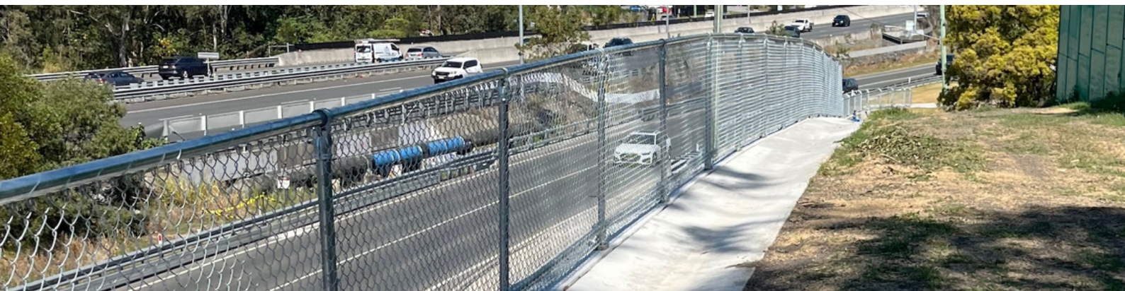
Fall protection chainwire on a road side
