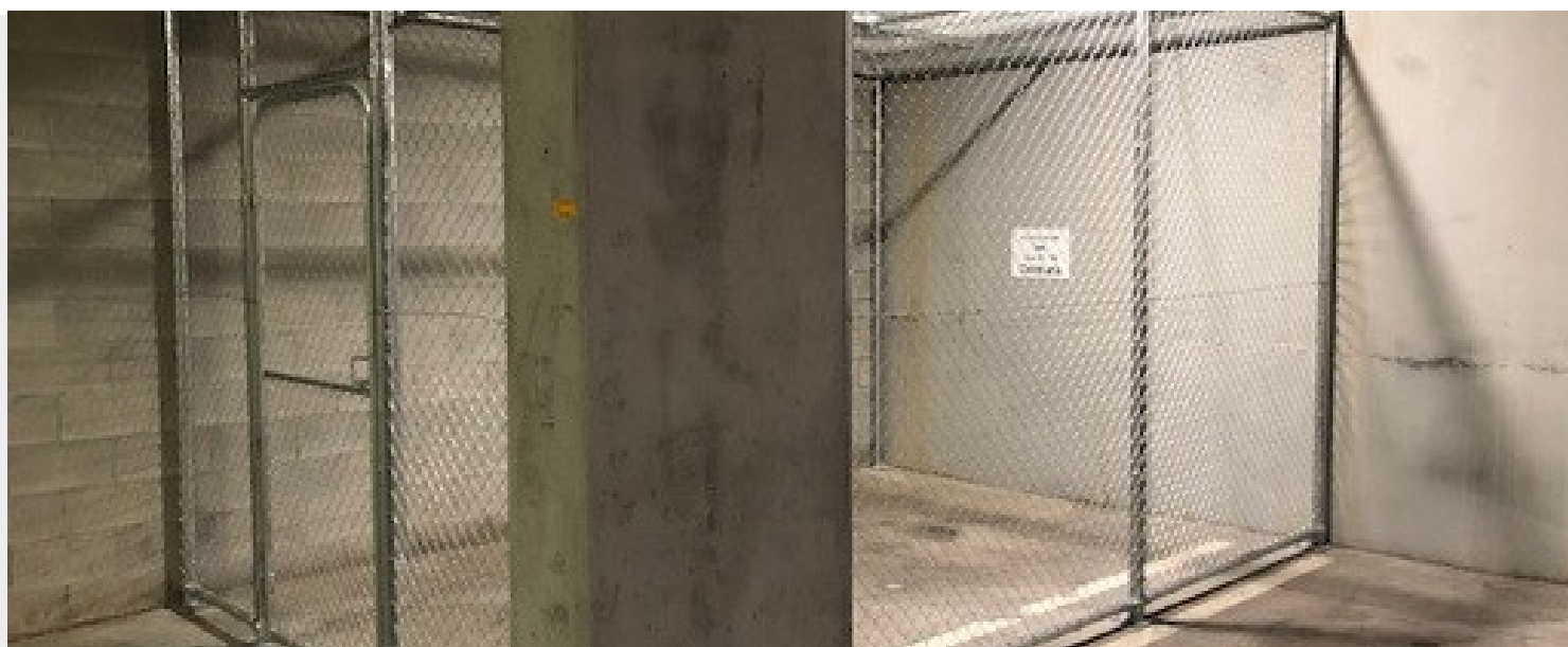
Galvanised Chainwire cage with single swinging gate in underground carpark
